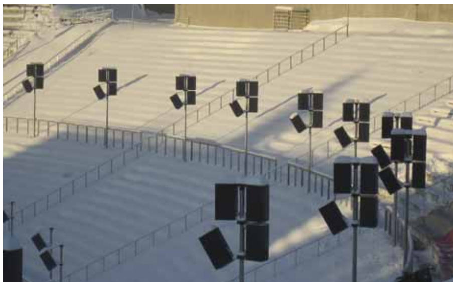
The Electro-Voice loudspeakers provided a convincing sound reinforcement solution without obstructing lines of sight for the TV cameras
