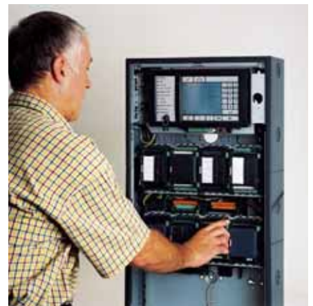
Modules of fire alarm control panel
